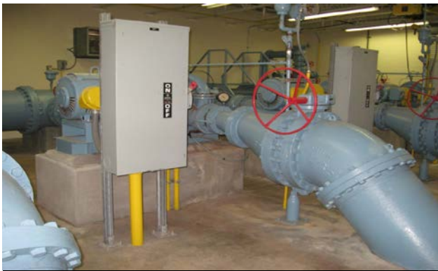
Equipment at Crossroads Booster Station
