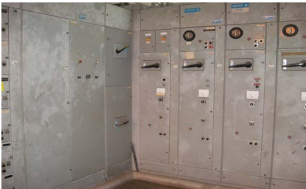
Electrical gear at the I & D Plant
