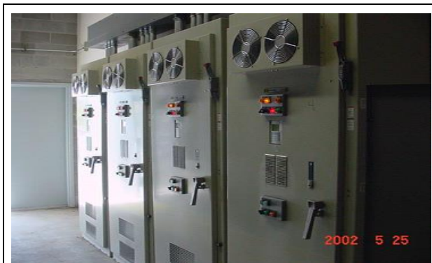
Current variable frequency drive equipment at plant
