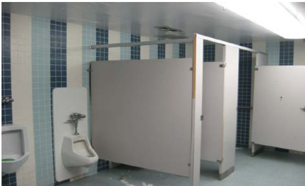
Civic Center restrooms in need of renovation
