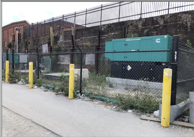
Typical Lift Station (W River Str - LS 72) SAVANNAH savannahga.gov
