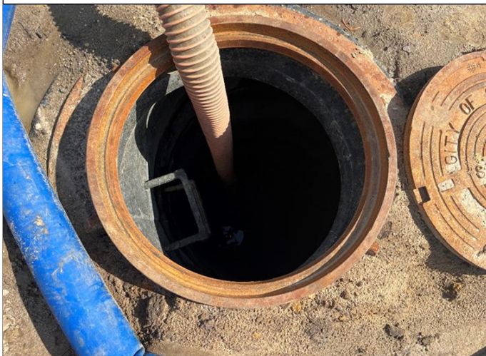
Water Valve Manhole
