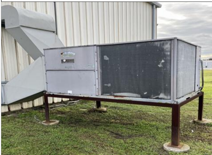
Aging HVAC Unit
