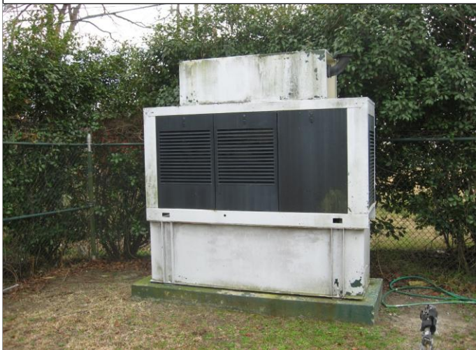
Aging Lift Station Generator
