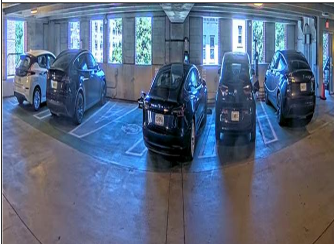
EV Charging Stations Bryan Street Parking Garage
