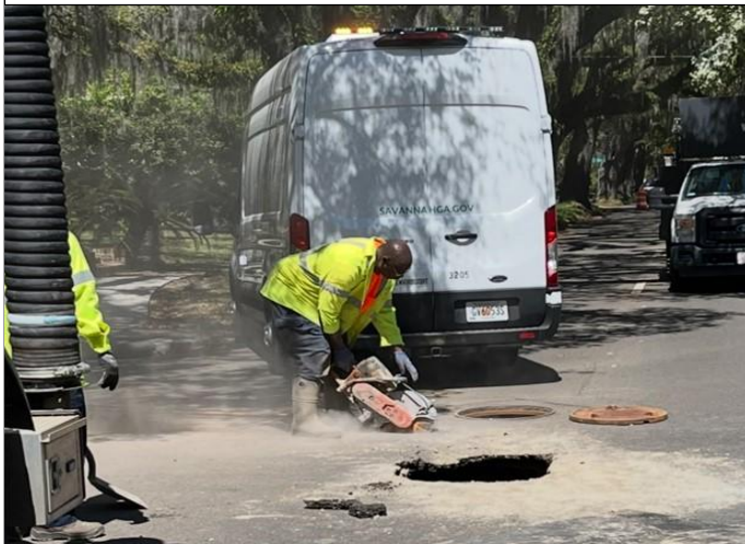
Abercorn Street Cave-In Repair
